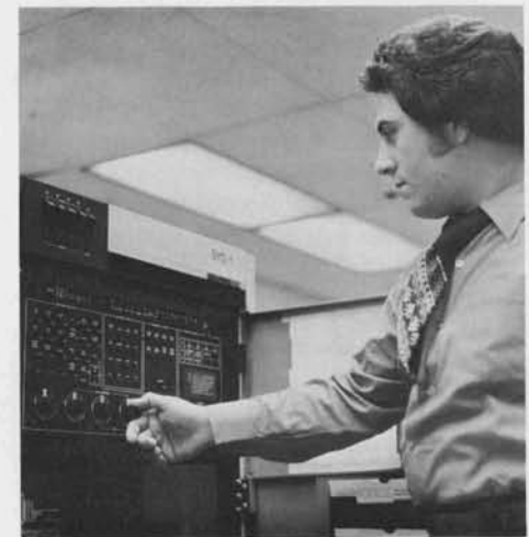
Trouble shooting a 3672 Controller at the Field Engineering Education Center in Santa Clara is John Crescenzo of the New York Island Branch Office.
